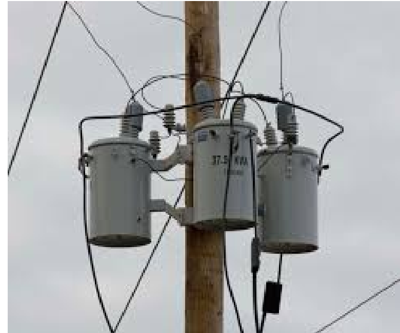
Three-phase transformer bank
